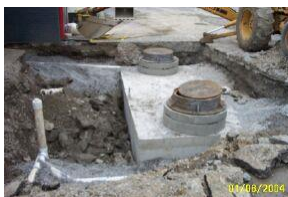
Grease Interceptor- surface views
